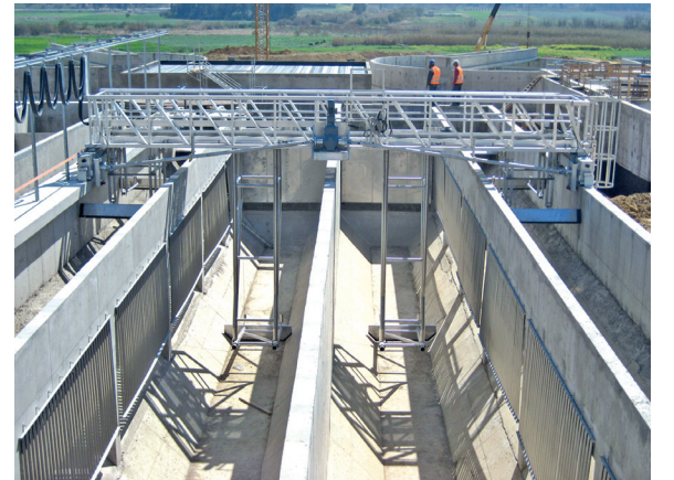
Grit & Grease Removal Scraper with Aluminium Truss Bridge
