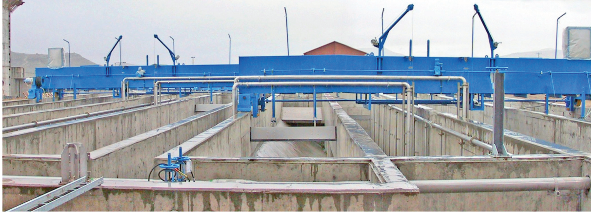
Travelling Grit Scrapers with grease skimmer blades
