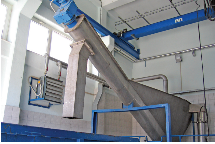
Grit Separator during operation
