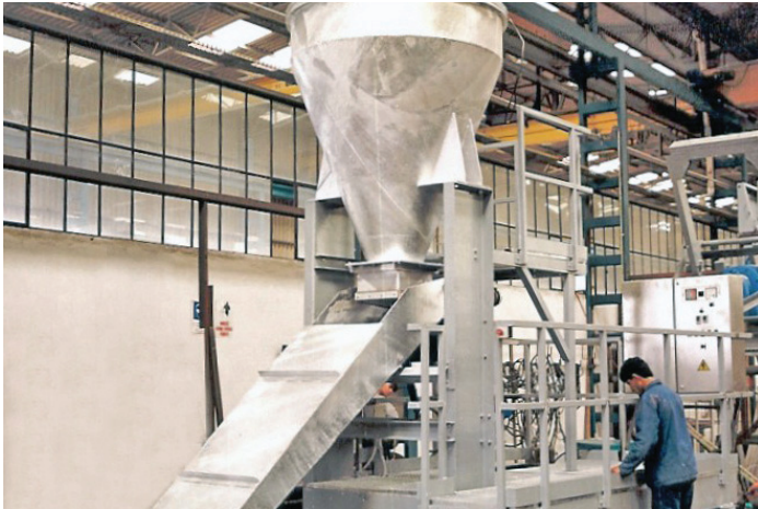
Grit Cyclone with Travelling Grit Scraper Bridge
