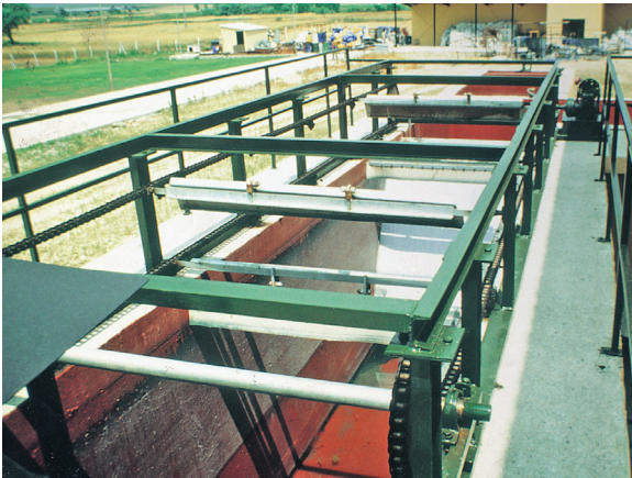
Chain Driven Surface Skimmer for Grease Removal
