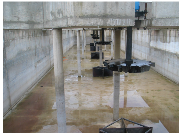
Vertical Shaft fixed type Turbine Aerators
