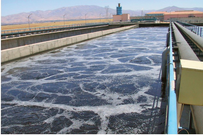
Diffuser Type Aeration System during operation
