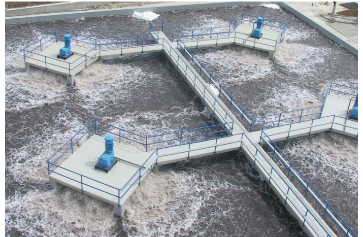
Vertical Shaft Turbine Aerators in operation
