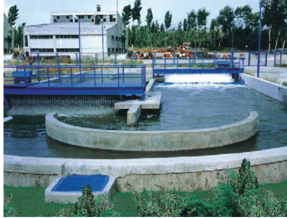
Horizontal Brush Aerators during operation
