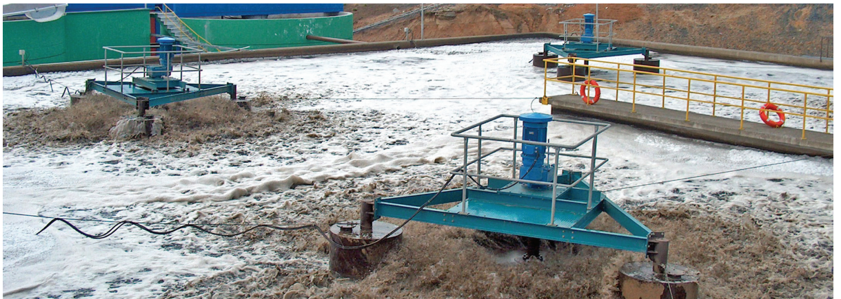
Vertical Shaft Turbine Aerators on floating pontoons during operation
