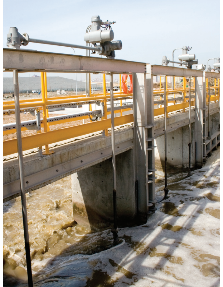
Weir type Penstocks with electrical actuators
